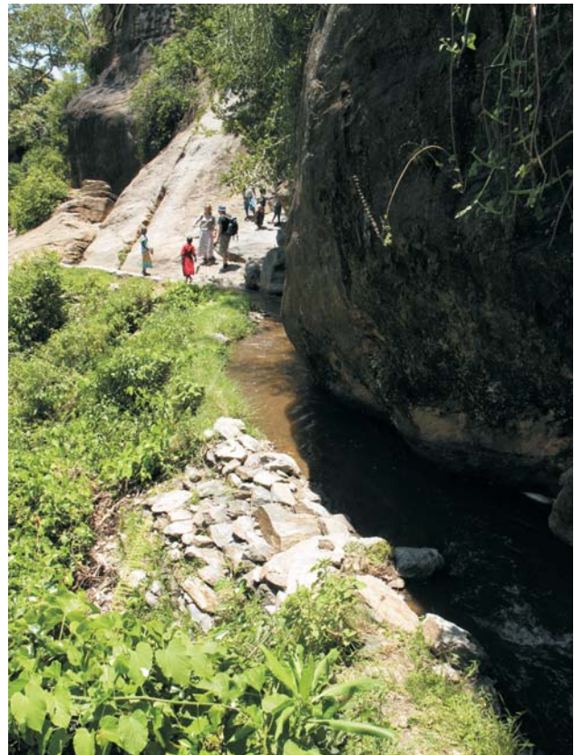
Fig. 3: A canal on a raised embankment in Marakwet. The stone-work in the foreground shows a patch of recent repair that will soon be covered by vegetation.
